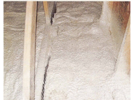
A This foam has pulled away from the truss chord due to excessive exothermic heat. Closed-cell foam should be installed in lifts that measure less than 2 inches thick, and with enough time between lifts to allow exothermic heat to dissipate.
