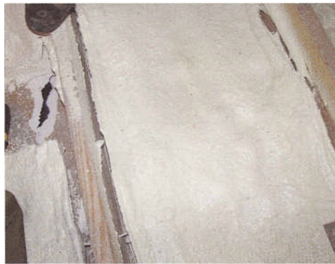
I Closed-cell foam was sprayed too thickly into this stud bay and has shrunk away from the framing as a result of exothermic heat build-up. The foam should be removed and replaced.
